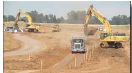
Trucks and excavators move dirt from Fancher Creek Detention Basin at McKinley and McCall for use in the Caltrans 180 East expansion project.
