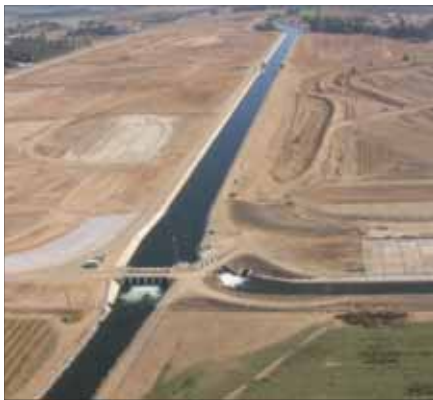
Looking east - channel branches off into Fancher Creek (l) and Mill Ditch (r) at the new head works.
